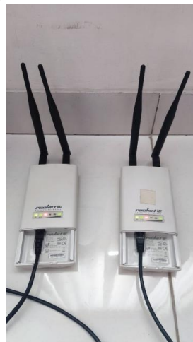
Figure 2 Access point for WMN
